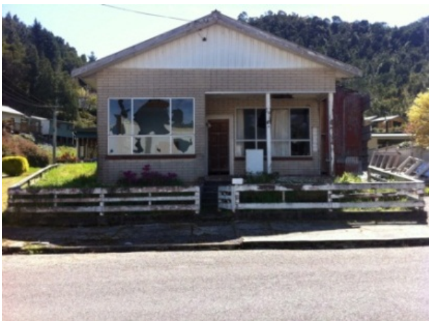
Figure 1: Building shows signs of dilapidation by way of broken windows and damaged exterior surfaces
