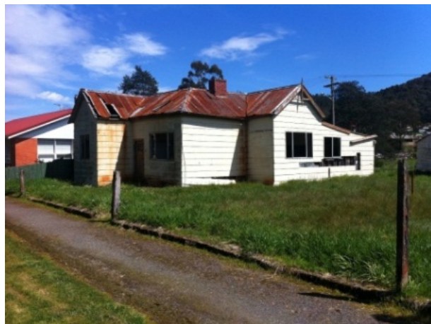
Figure 2: Building shows signs of dilapidation particularly compared to the neighbouring house
