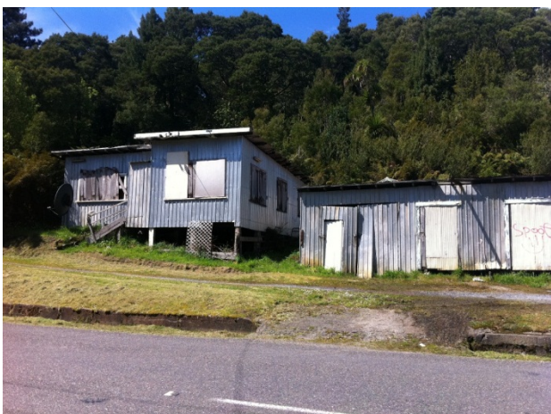
Figure 3: Building shows signs of dilapidation by way of damaged exterior building surfaces and graffiti. Building may also have structural defects that, if unfit for use or occupation, or a danger to users of the building, can also be addressed through the building notice/order process under the Building Act.
