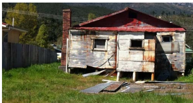
Figure 4: Building shows signs of dilapidation by way of damaged exterior building surfaces and damaged roof coverings. Building may also have structural defects that can also be addressed through the building notice/order process under the Building Act.
