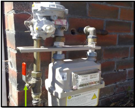
Gas supply valve on
