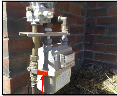
Gas supply valve off
