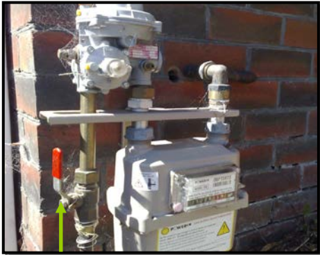
Gas supply valve on
