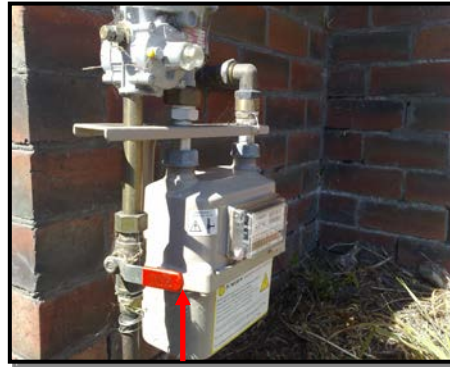
Gas supply valve off
