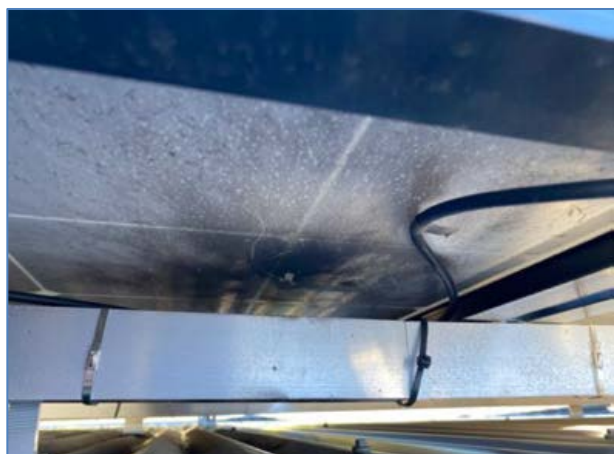
Result of a poor crimp under the array
