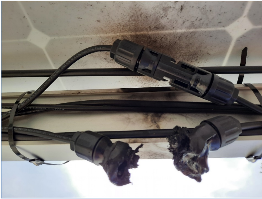
Example of failed mismatched d.c. connector
